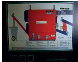
↑ PCT 400 control screen
