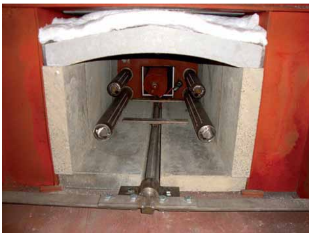
↑ View of the refractory hearth with primary and secondary stainless air nozzles. Scraper for ash removal and to assist in clinker break up
